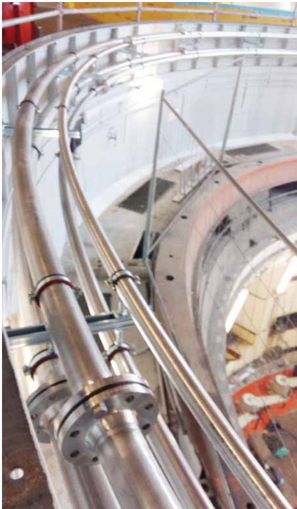
Kühlwasserverteilung | Cooling water distribution
