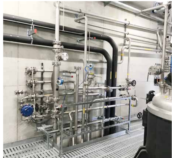
Chemieverrohrung | Chemical pipe installation
