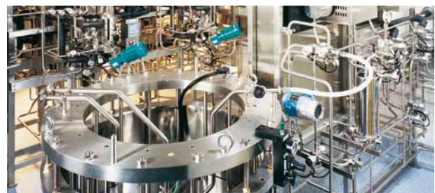
Reinraummontage | Clean room assembly
